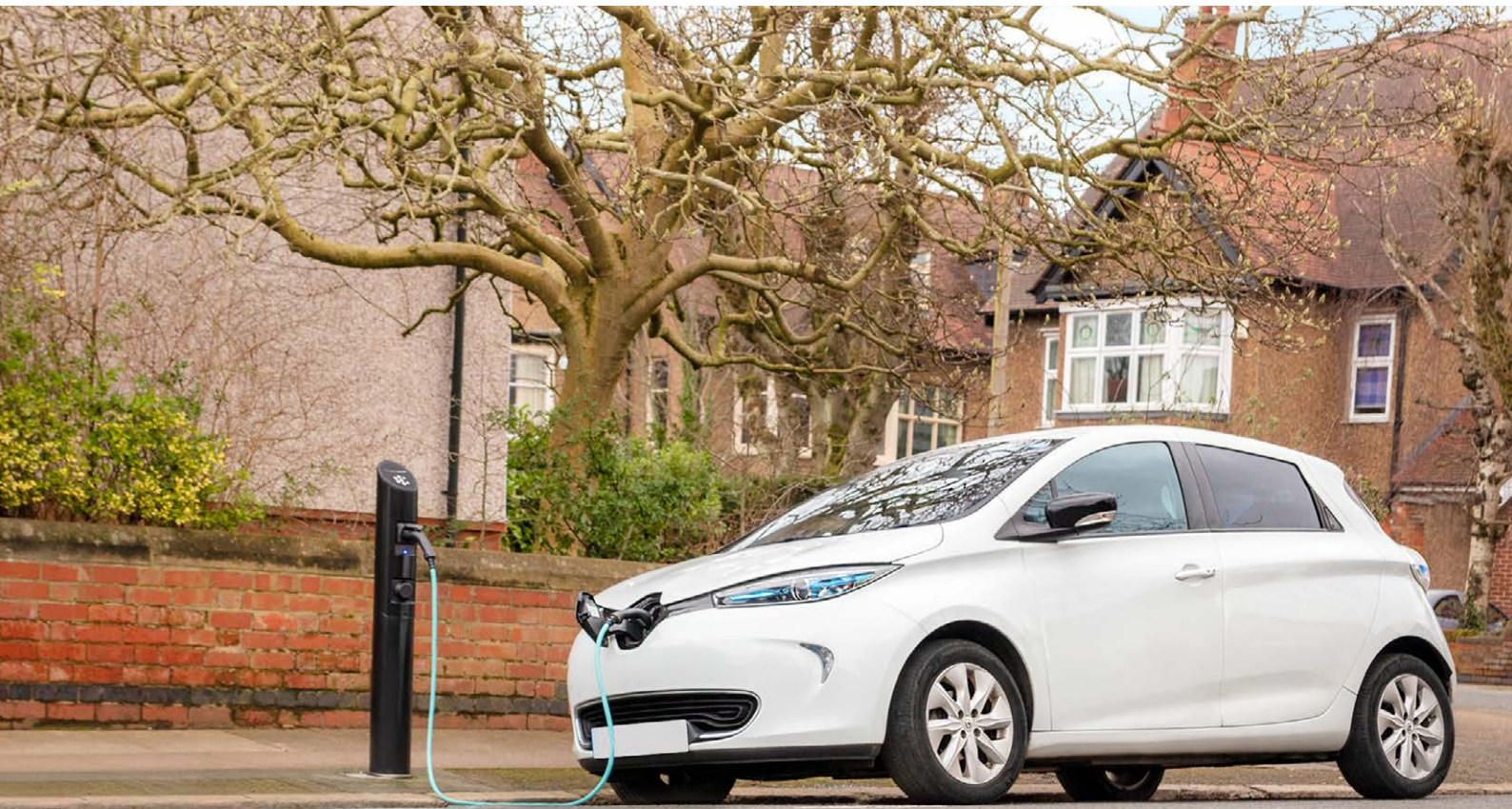
A charging bollard feeding electricity off a lamppost at the back of the pavement
