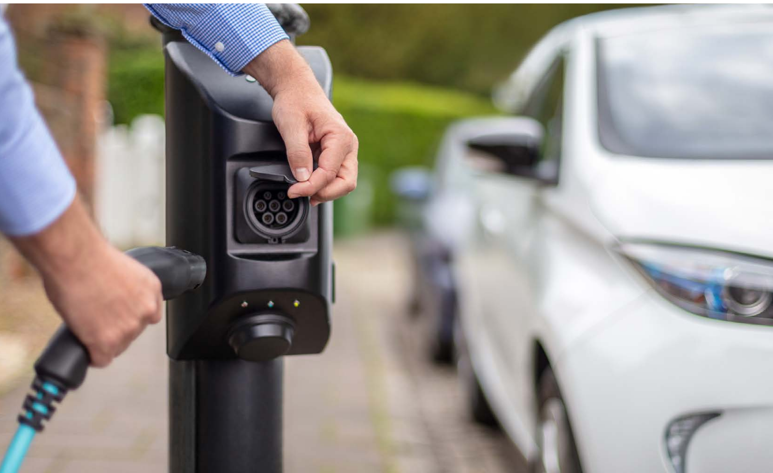
The chargers are housed in lampposts
